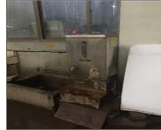
Photo of the sanitary facilities 13-1 Potable water.JPG
